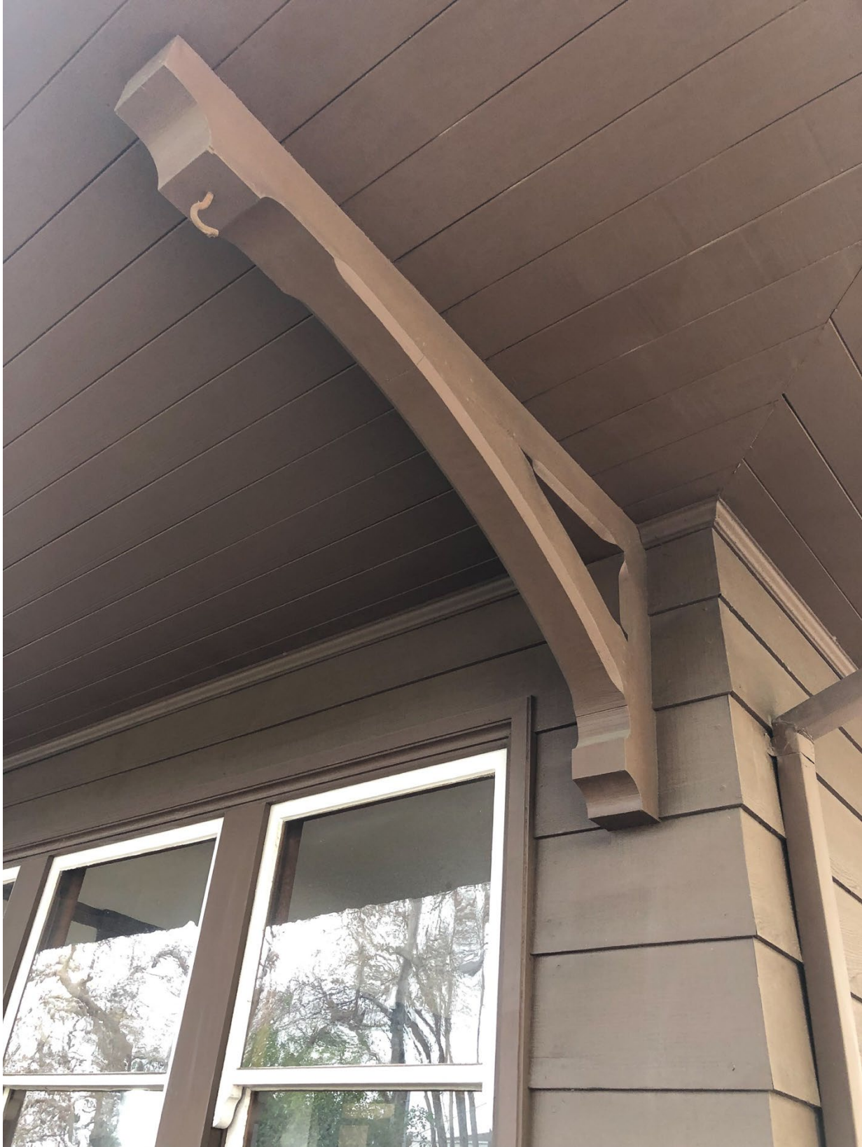
Fig.18 – 2119 Marin Ave. – Bracket at front porch
